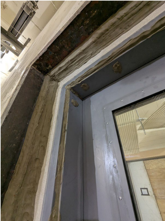
Figure 6 – Detail of mastic on door frame on receive room side
